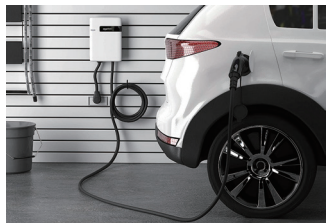
Electric Car / Fast Charging
